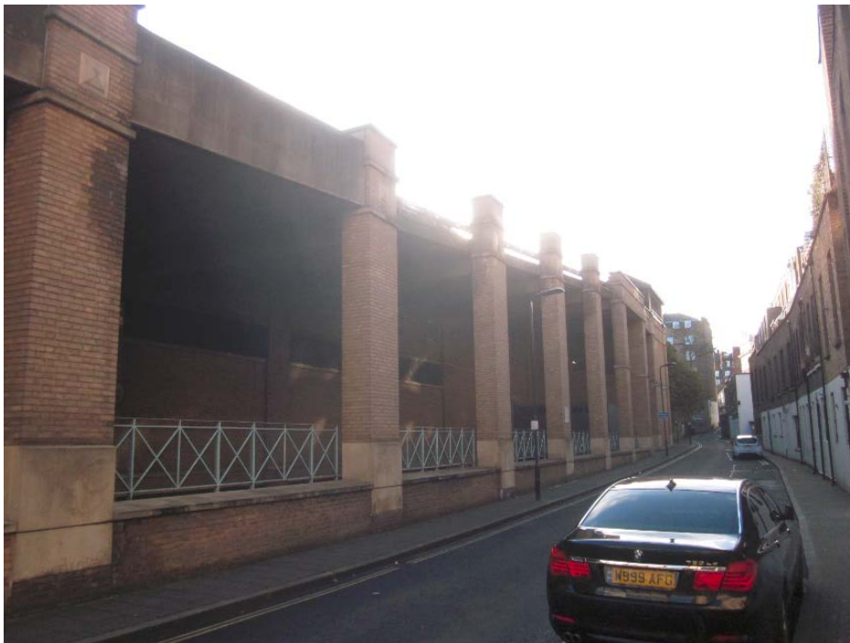
Front (west) elevation at corner of Queensway and Porchester Gardens (top) and rear (east) elevation in Redan Place (bottom).
